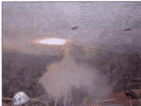
Figure 11. High-pressure Gas Emission from a Relief Hole in the Roof at OCI
