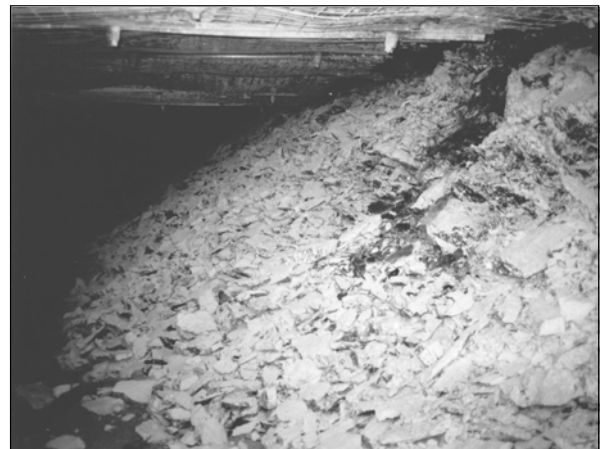
Figure 4. Full Yielding of a 9.1-m-wide Yield Pillar Under Tailgate Loading Conditions in the Book Cliffs Coal Fields
