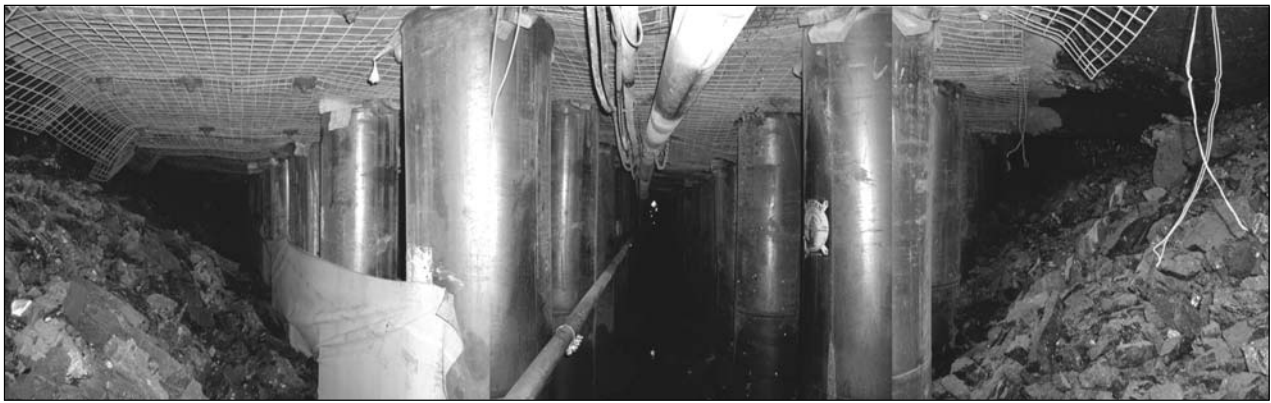
Figure 7. Typical Ventilation Return Ahead of the Front-abutment Zone with a Two-entry Yield Pillar Gateroad System
