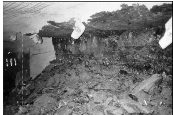
Figure 3. Aftermath of a 1-m-deep Rib Bump at the Corner of an Abutment Pillar
