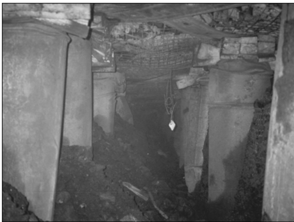
Figure 8. Heavy Convergence in the Tailgate Caused by Front-abutment Loading with a Two-entry Yield Pillar Gateroad System
