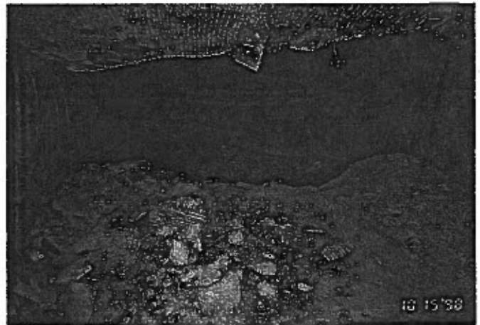
Figure 6a. Smooth Dome-shaped Roof Fall Across Laminated Strata in an Intersection
