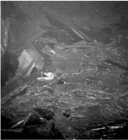
Figure 2. Large Roof Fall from Paleo-Channel
