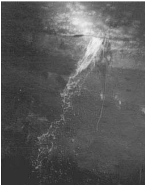
Figure 4. Water Emanating from Open Joint
